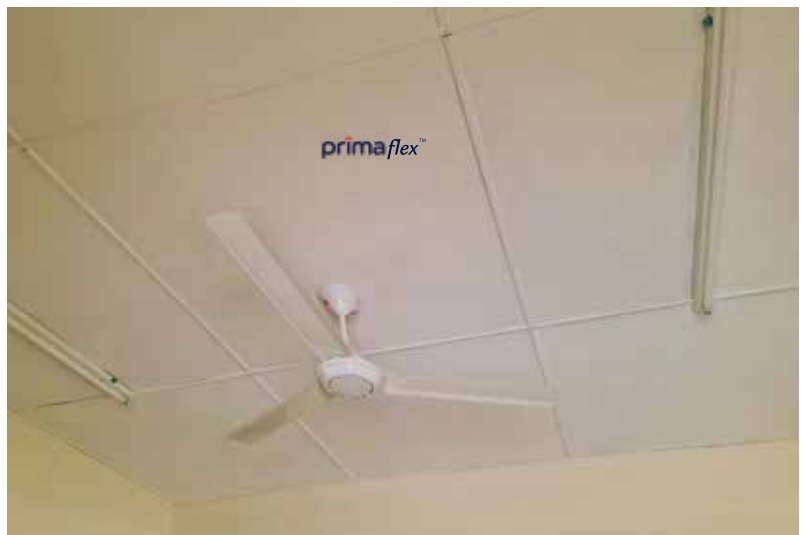
Fittings installed to the ceiling as per manufacturer's recommendation
