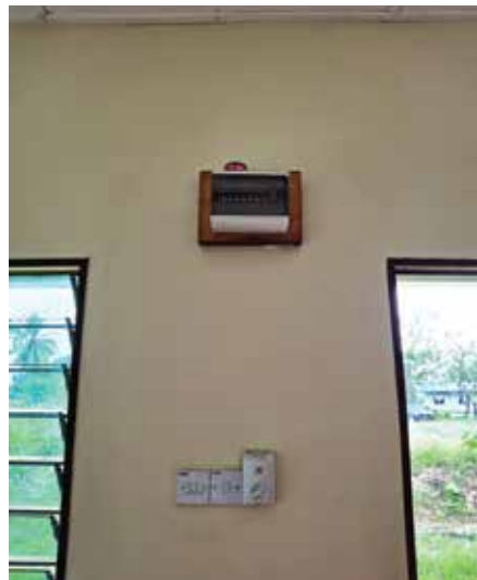
Wall switch and DB box on PRIMA Board
