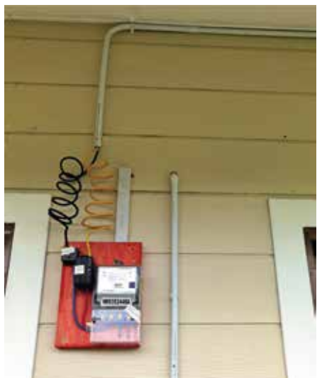
Main meter box installed on PRIMA IBS wall
