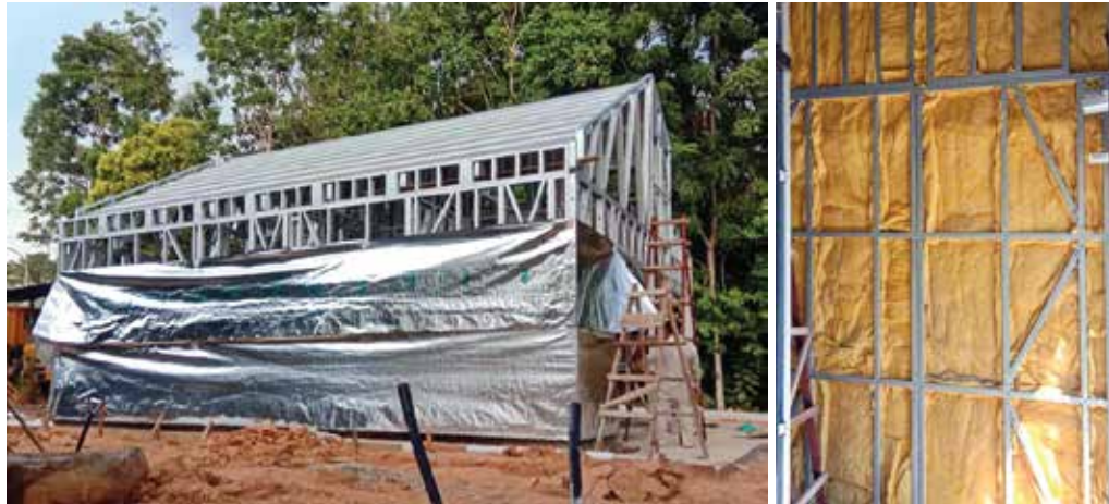
Sisalation sheets on LGS frames before install PRIMA fibre cement boards Wall insulation (optional)
